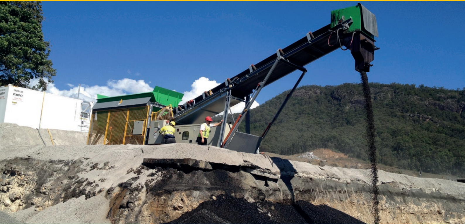
Plant producing pre-coated aggregate
