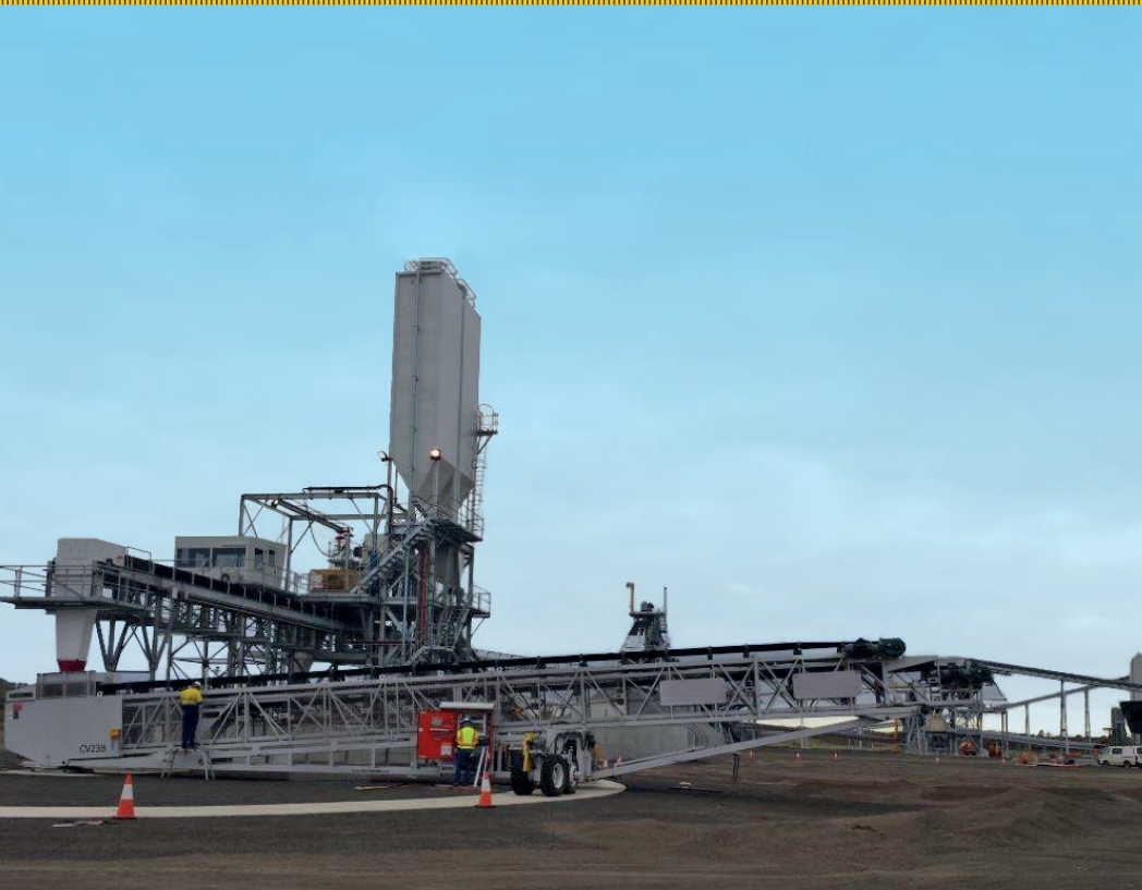
600 tonnes per hour cement treated base (CTB) plant
