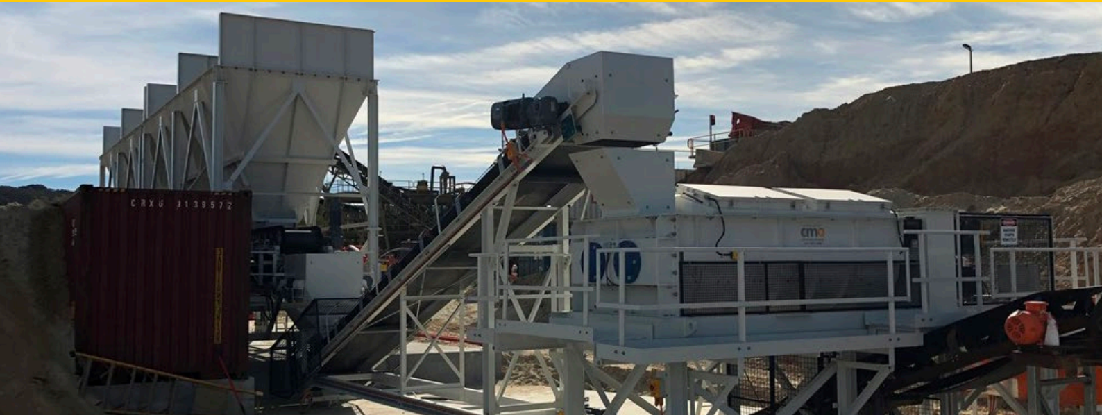
Sand blending plant with 4 belt weighers and receiving bins
