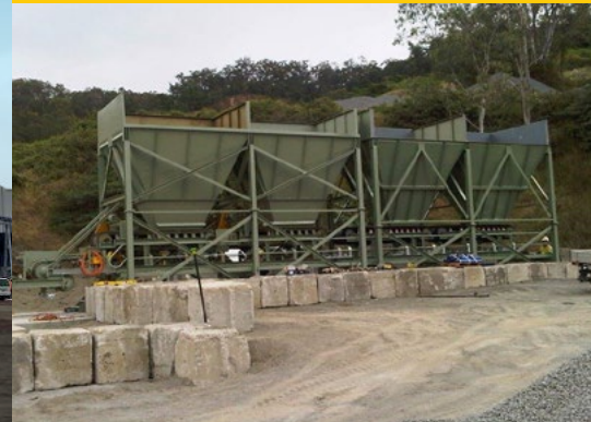
Receiving bins with belt weighers
