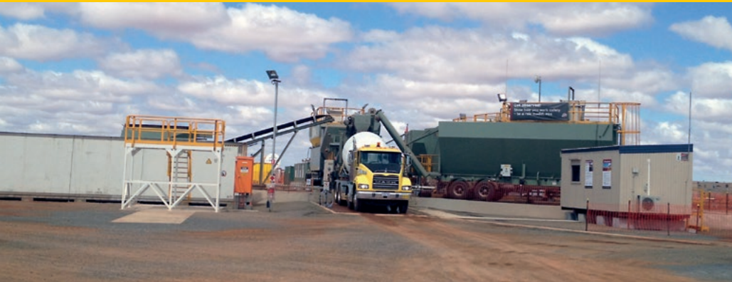
Mobile train arrangements Wheatstone Project WA 1 Portabatch, 3 x 75T mobile silos, 1 auxiliary weigh hopper
