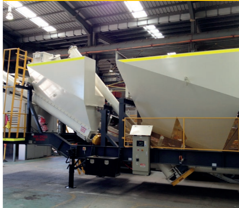
Cement weigh hopper filter access
