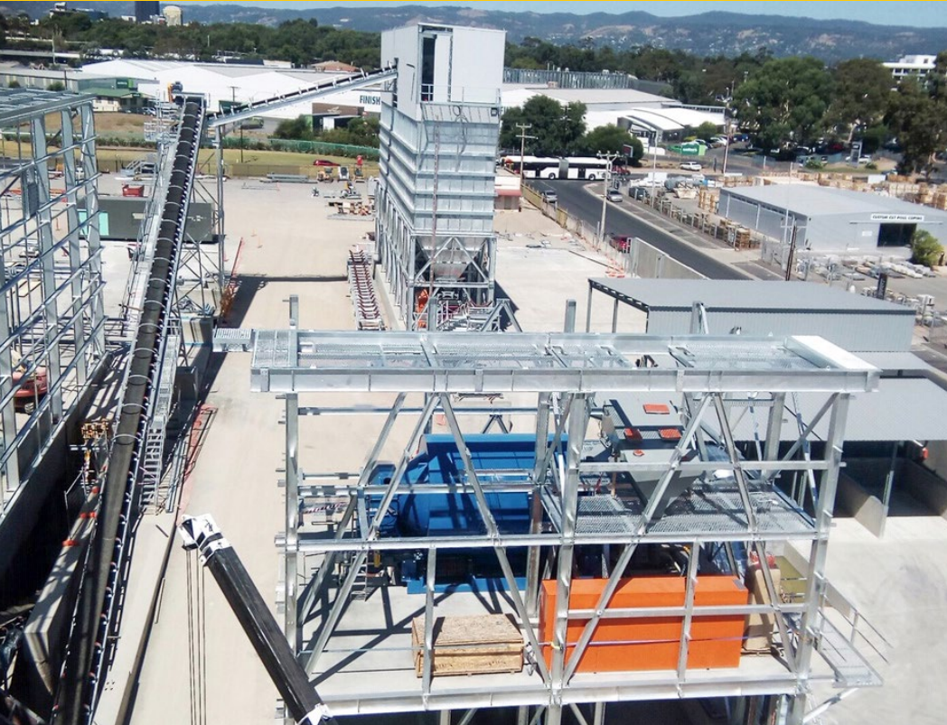
Wet mix plant 220m 3 /hr
