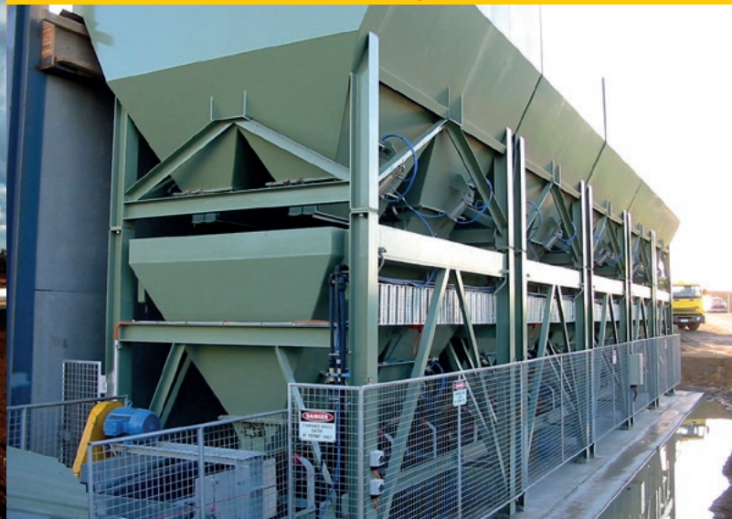
Aggregate receiving bins and weigh hoppers
