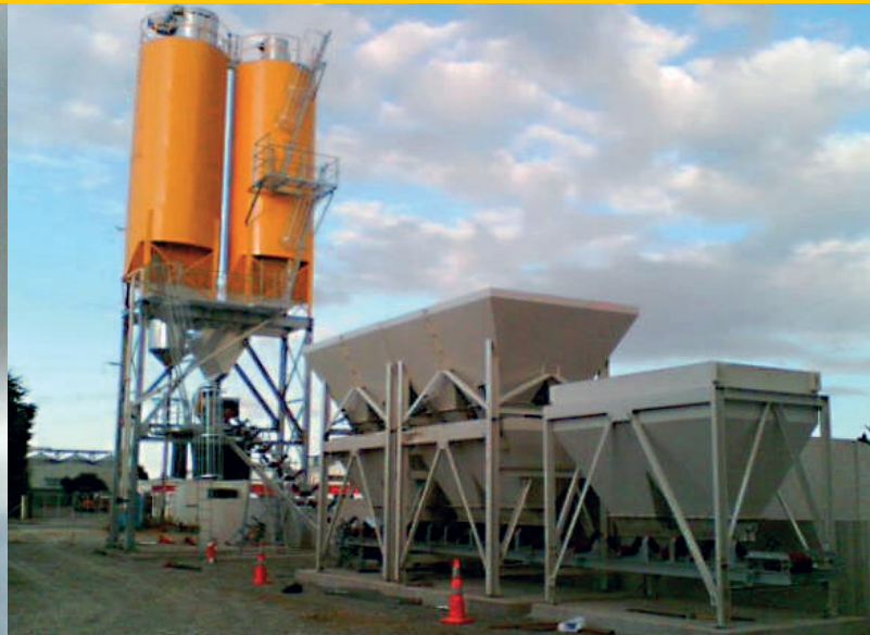
Front end loader fed plant with 2 x 22T 4-compartment spotting bins and a specials bin
