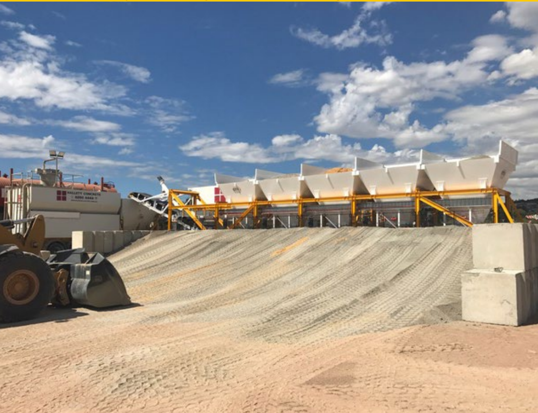
5-bin aggregate trailer with belt weighers
