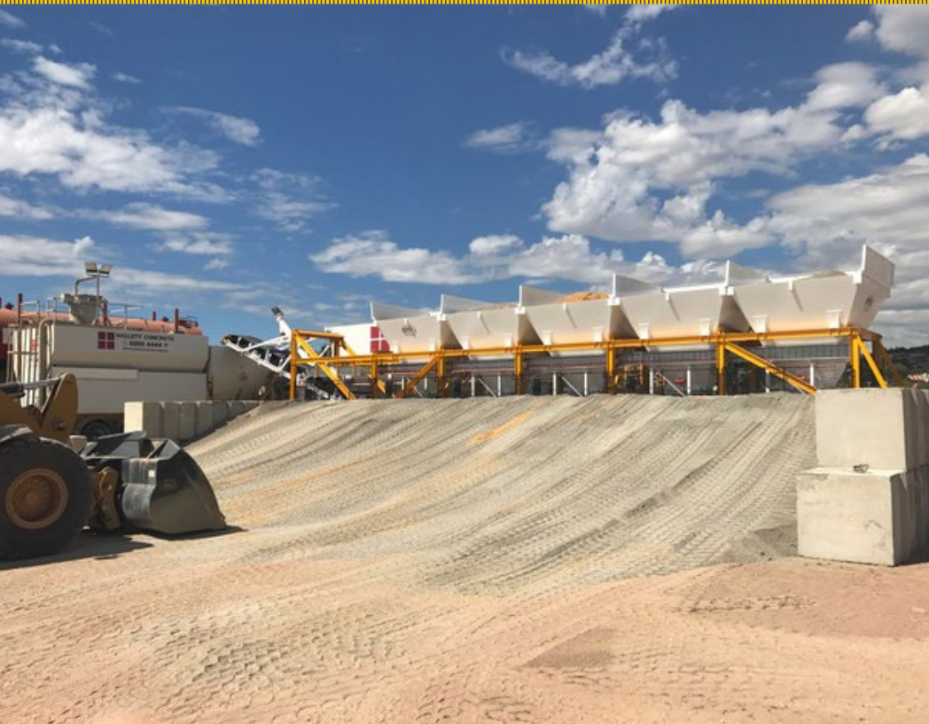
5-bin aggregate trailer with belt weighers
