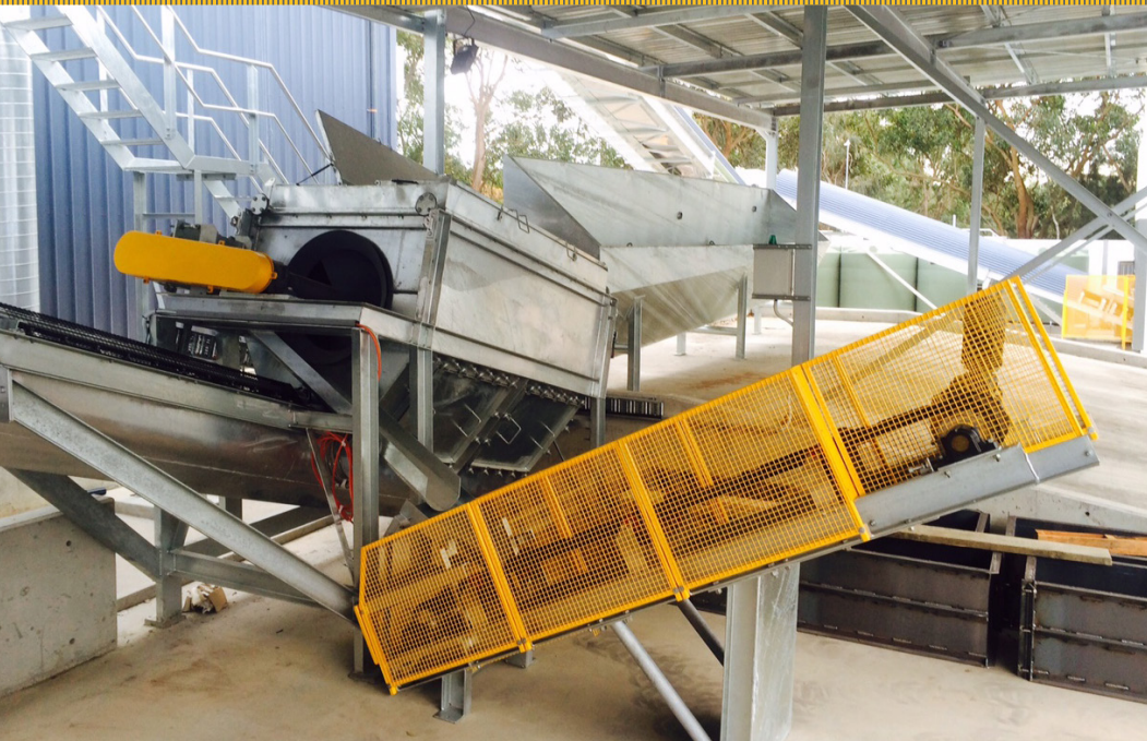
Reclaimer, truck wash out trough and conveyor
