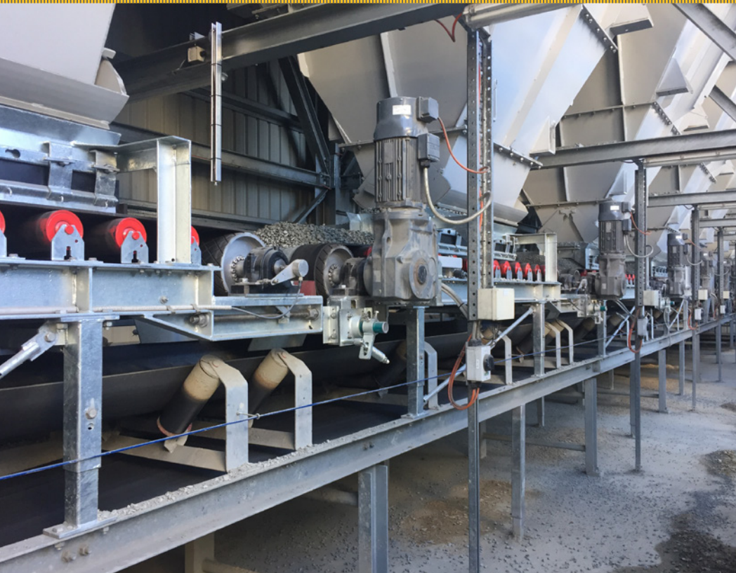
Typical belt weigher under a multi storage overhead bin
