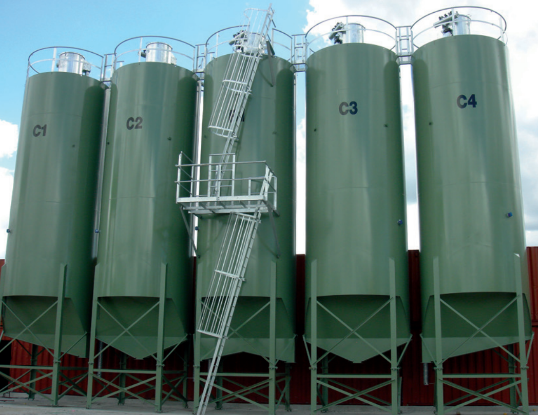
80T storage silos. Centre silo features dual outlet
