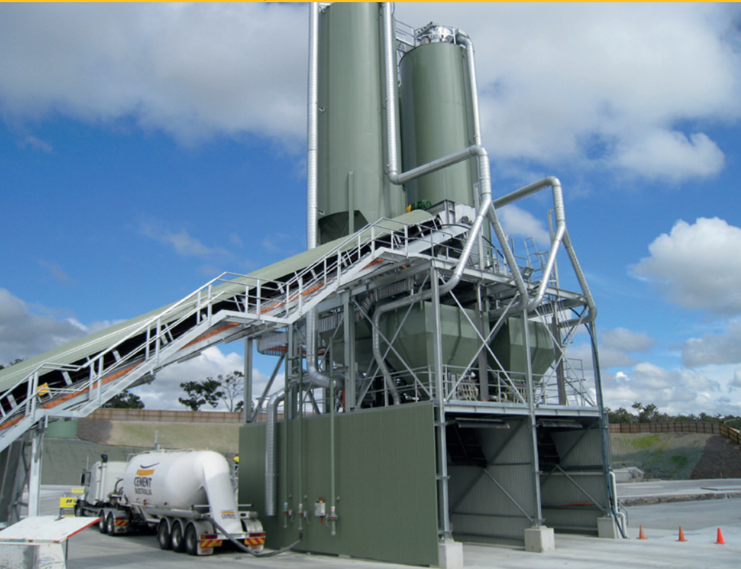
120T dual outlet cement colis feeding cement hoppers
