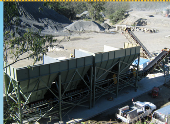
Blending plant with 4 bins
