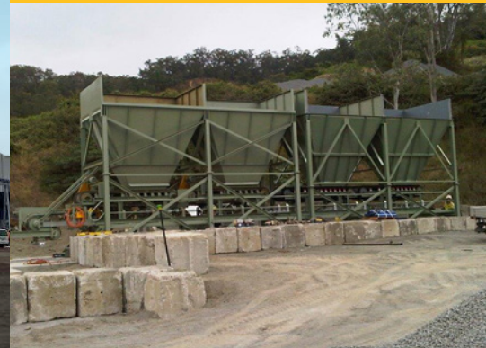
Receiving bins with belt weighers
