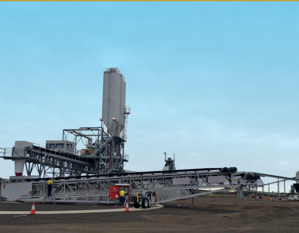
Cement treated base (CTB) plant
